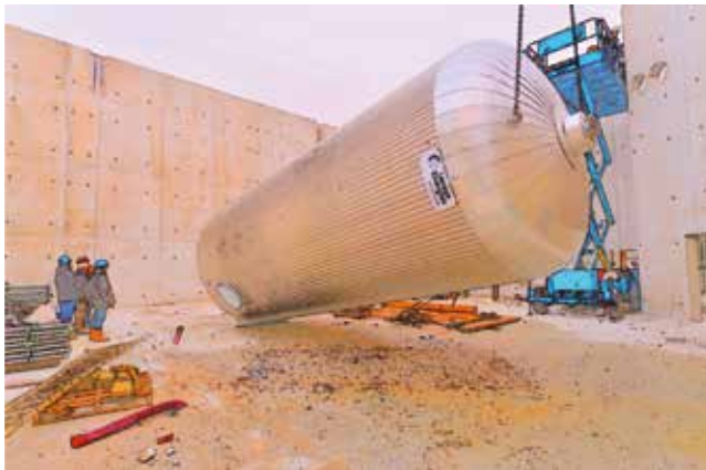
■ Ballon hydro-accumulation 2*60 m 3 - © ENB
