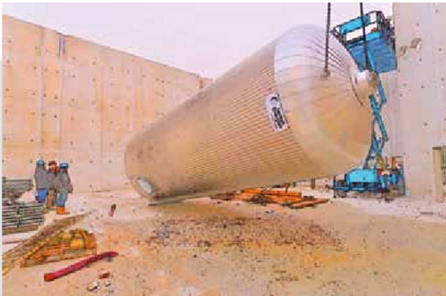
Ballon hydro-accumulation 2*60 m 3 chaufferie bois 2*2,5MW Bacalan Bordeaux (33)
